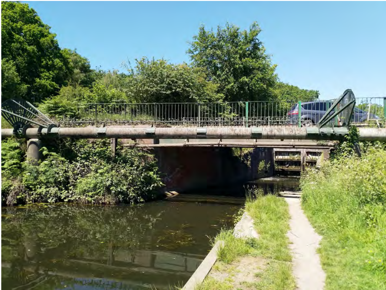
Image 25—View Looking North West towards Government Road Bridge and Ash Lock beyond
